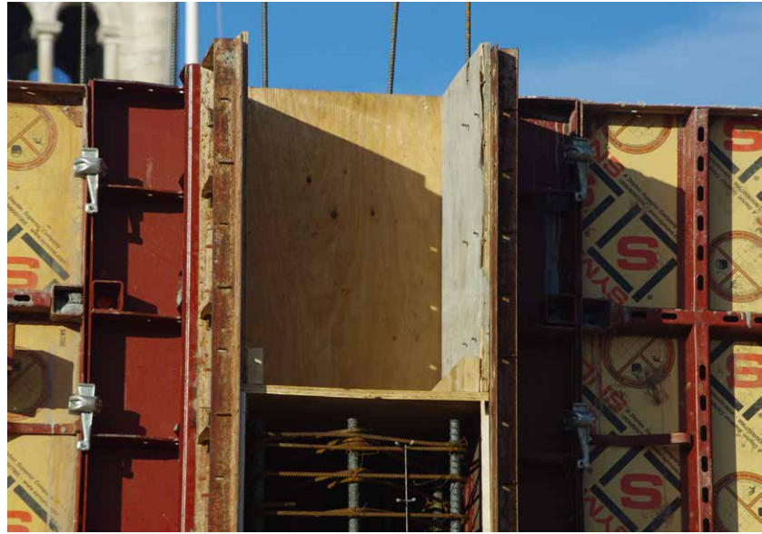
The contractor was able to gain boxout access by using Steel-Ply on at least one face of every pilaster because of its compatibility with Sym-Ply.
