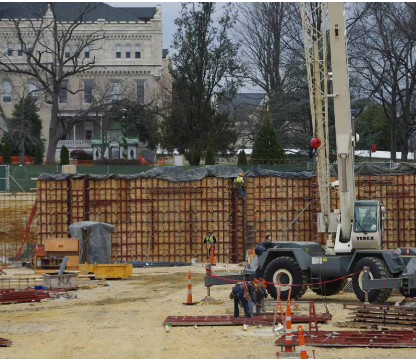
Ganging forms allows contractors to position large blocks of forms at a time, speeding set-up and take-down procedures.
