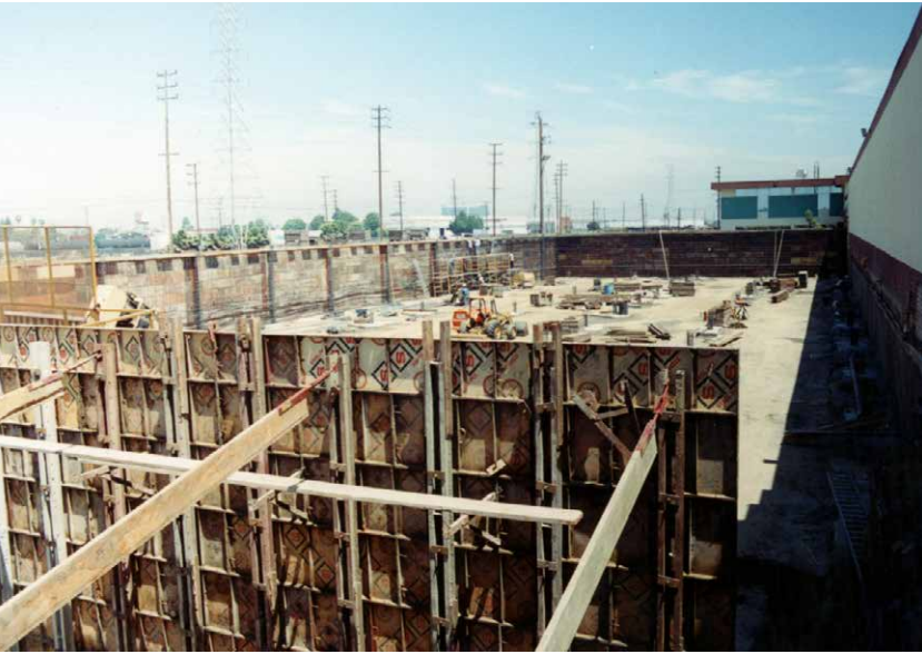
This project incorporated horizontal Steel-Ply gangs in combination with handset pilasters and corners for a productive system.
