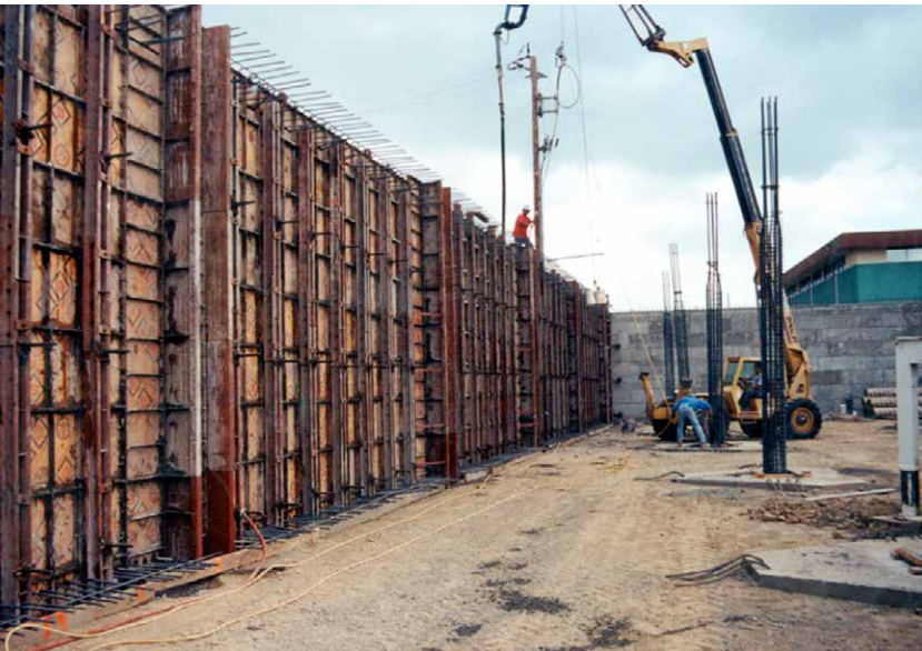
Pilasters were handset between the gangs of horizontal Steel-Ply, providing the contractor with gangform productivity and handset versatility. Steel-Ply accommodated the rebar penetrations required for tying into subsequent floor and ceiling pours.
